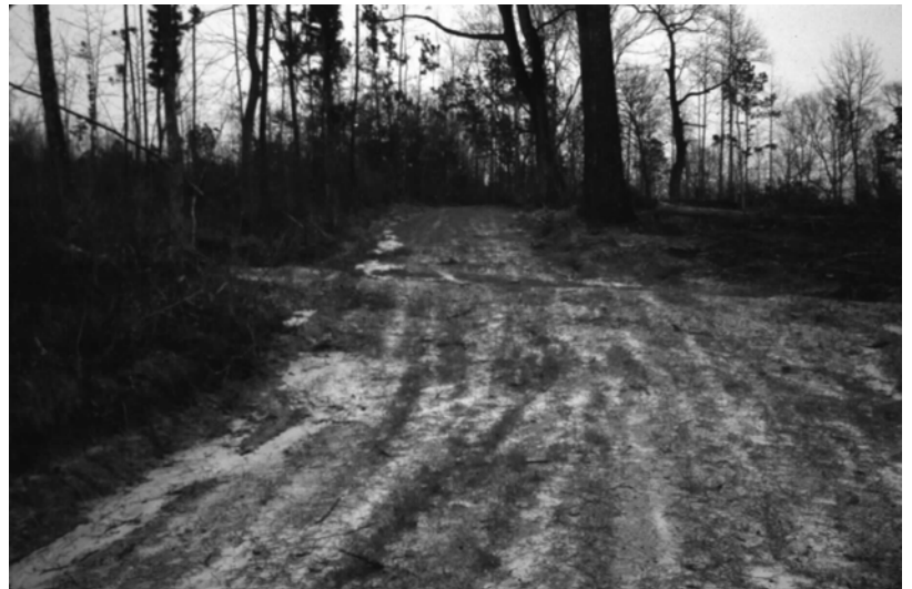
A firelane such as this needs water control structures to minimize erosion.
