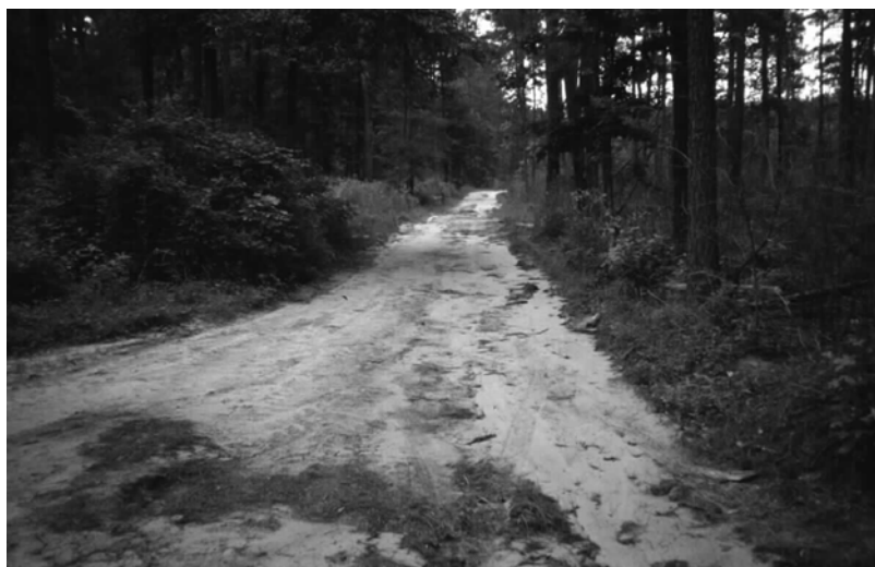
A washout like this can result from failing to maintain the road ditch and wing ditches.
