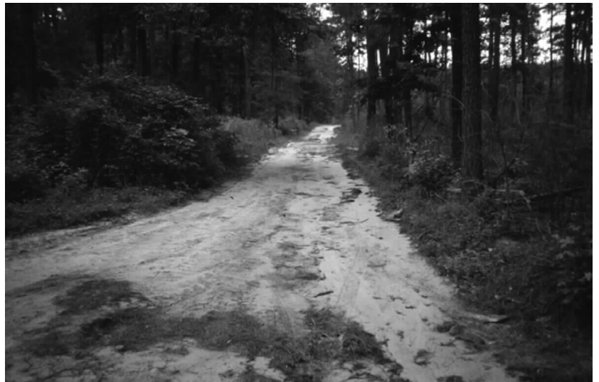
A washout like this can result from failing to maintain the road ditch and wing ditches.
